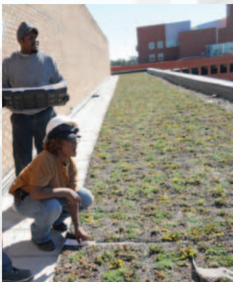
Chelona Bates and Augustus Brown work on the roof of the Warren Police Department after completing the Green Roof Installer Certification Course offered at Macomb's South Campus this summer. All 14 students who completed the course were hired by Newton Crane Roofing, Inc. to install green roofs on buildings in Warren's municipal complex.
