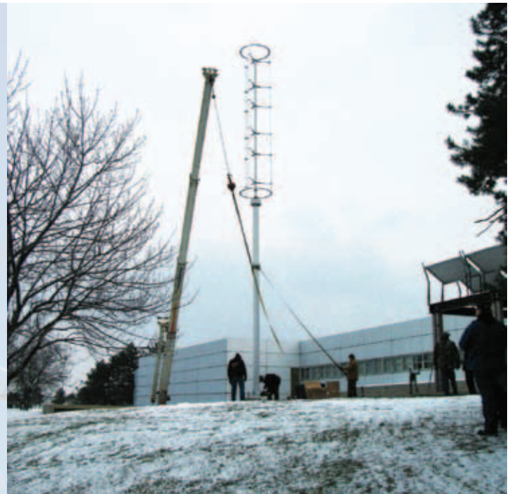
Workers install a wind spire on South Campus, which supports student studies in renewable energy.
